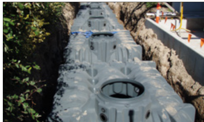
30,000 l (7,926 US gal.), Industrial plant, Geelong (Australia)
