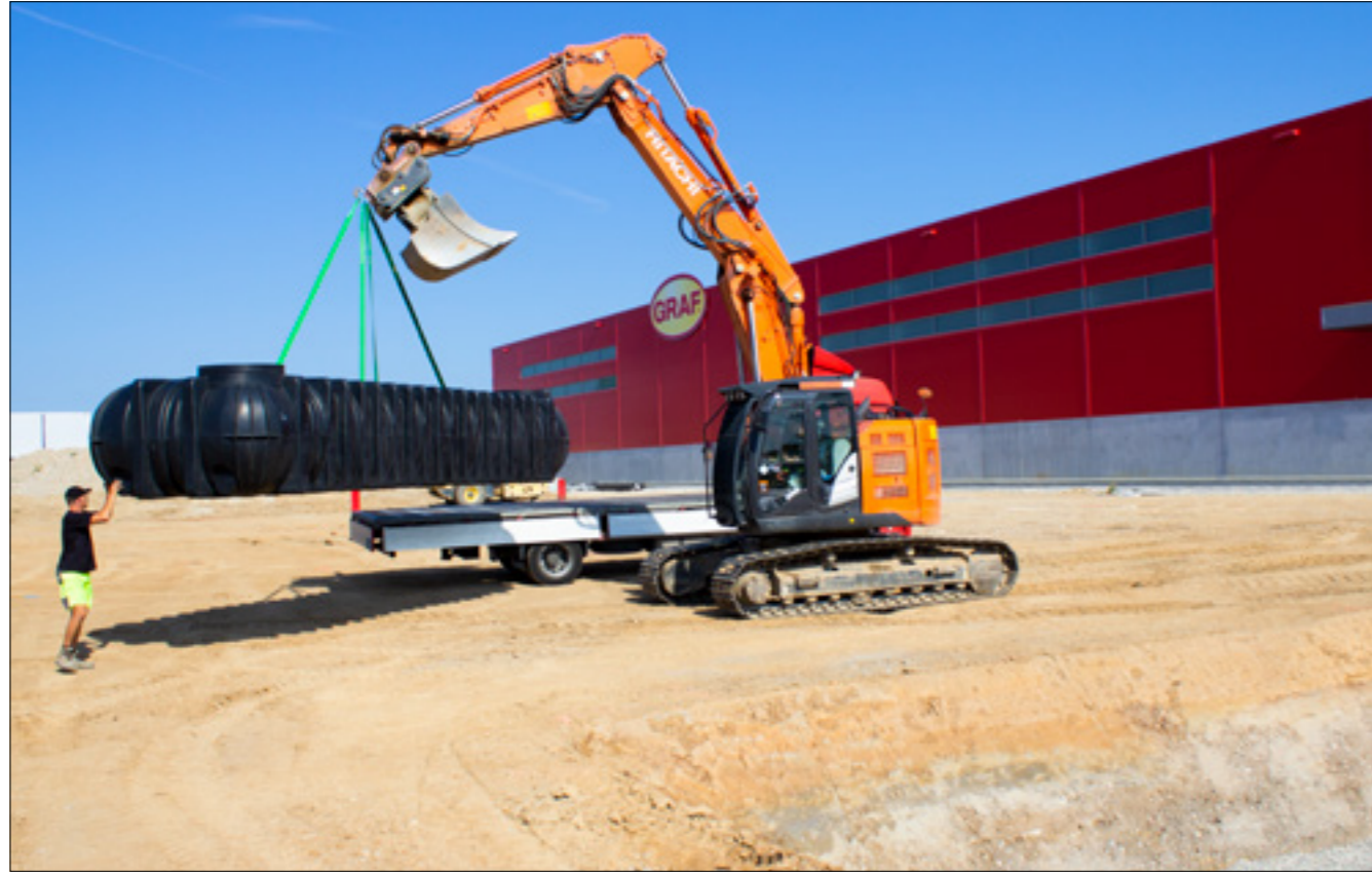
15,000 l (3,960 US gal.), Production plant, Herbolzheim (Germany)
