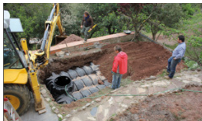
3,500 l (925 US gal.), Building, Vacarisses (Spain)
