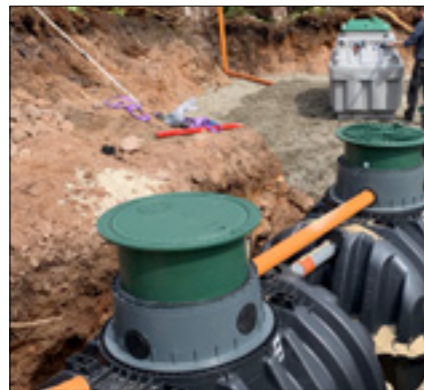
10 PE one2Clean with pumped Outlet, County Mayo
