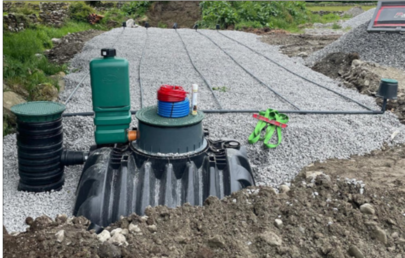
7 PE one2clean with 90 m 2 Low Pressure pipe distribution Co, Galway
